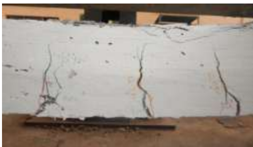
Figure.7 Typical crack pattern of Beam
