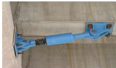
Typical anchoring configuration of a fluid viscous device (photo taken during the installation).
