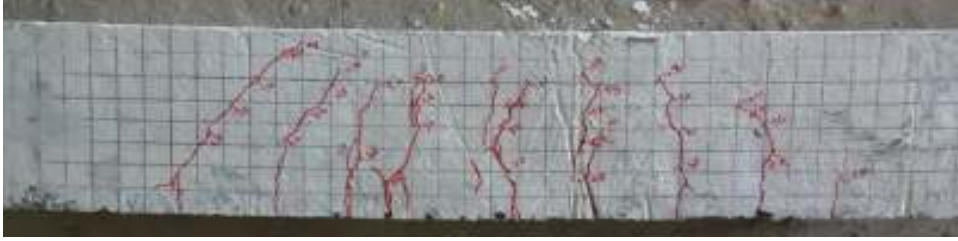
Fig.7 Crack pattern of W-3
