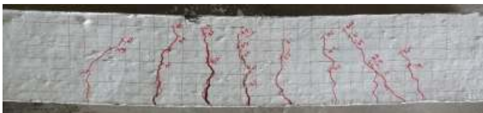
Fig.6 Crack pattern of W-2
