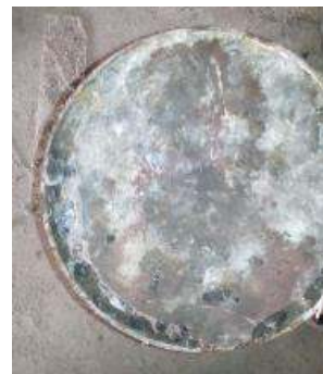
Figure 7: Failure in bond
