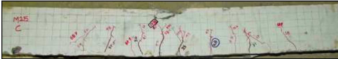
a. Crack pattern for M25 control beam
