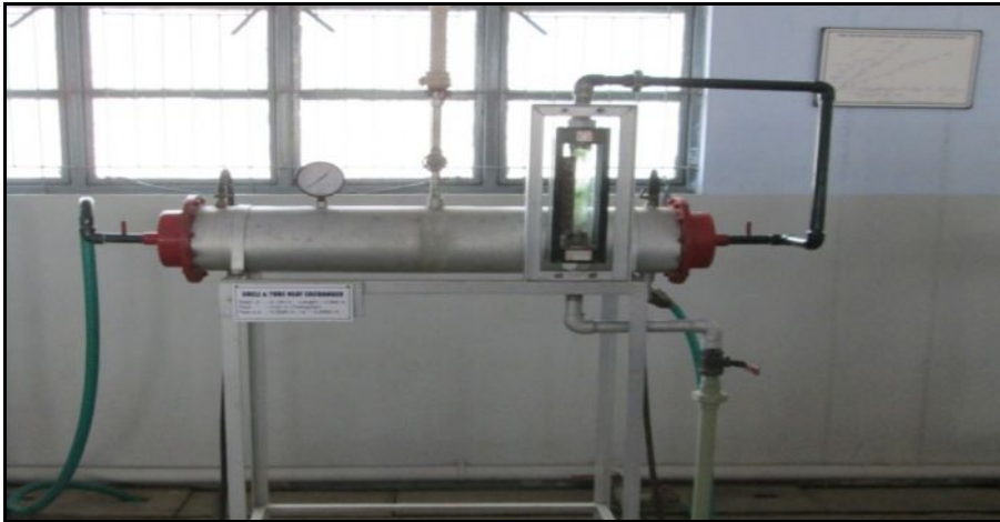
Figure. 1 Real Time Setup of Shell and Tube Heat Exchanger
