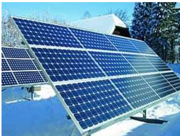
Figure 3 : Installed PV array
